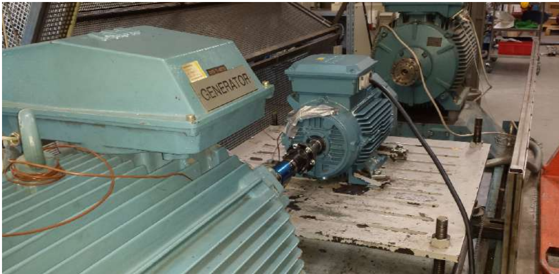
Motor test facility, M-Lab - Danish Technological Institute, Taastrup
